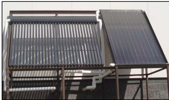
Solar hot water heating at Badger State Inc.
